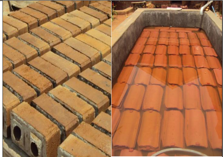
Above: Both ISSBs and Concrete roof tiles above on the left and right respectively under curing stage before use
